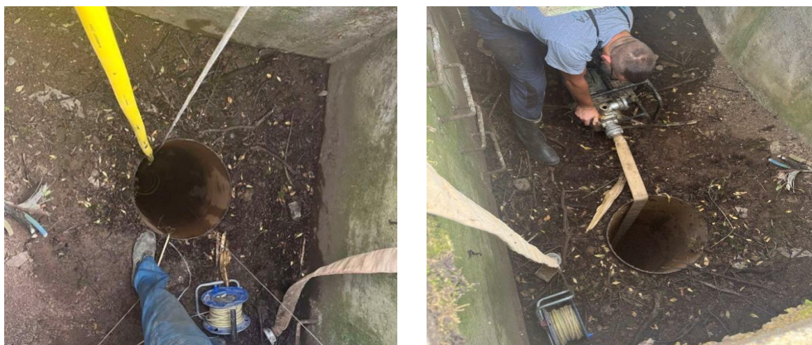
Figure 35. Performing pumping tests on the subject well and monitoring GWL on neighbouring wells
